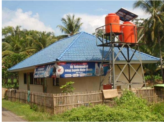
A newly installed solar operated well
